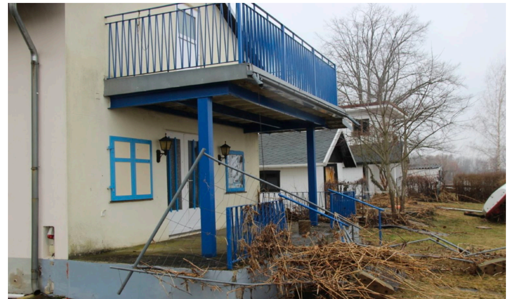
Damage caused by the displacement wave at Knappensee in Germany. Image by Torsten Richter-Zippack via LR Online .
