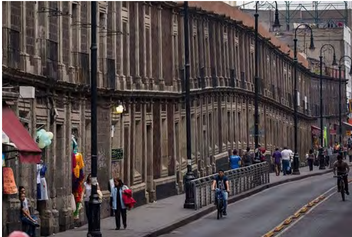
Mexico City's buildings are seriously leaning due to land subsidence. Photo credit: JOSH HANER/THE NEW YORK TIMES ( http://www.sciencemag.org )
